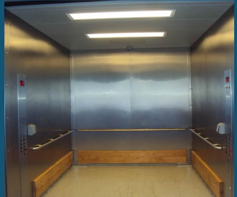
Central Terminal Freight Elevator #2
